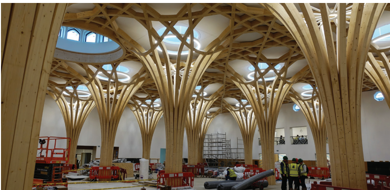
The eco-mosque has 30 Free Form timber columns that support and sprout into the lattice roof.
