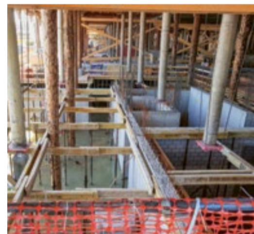
The Kornhaus was completely gutted during conversion. Around 80 tree trunks carried the weight of the building in the first phase of renovation.
